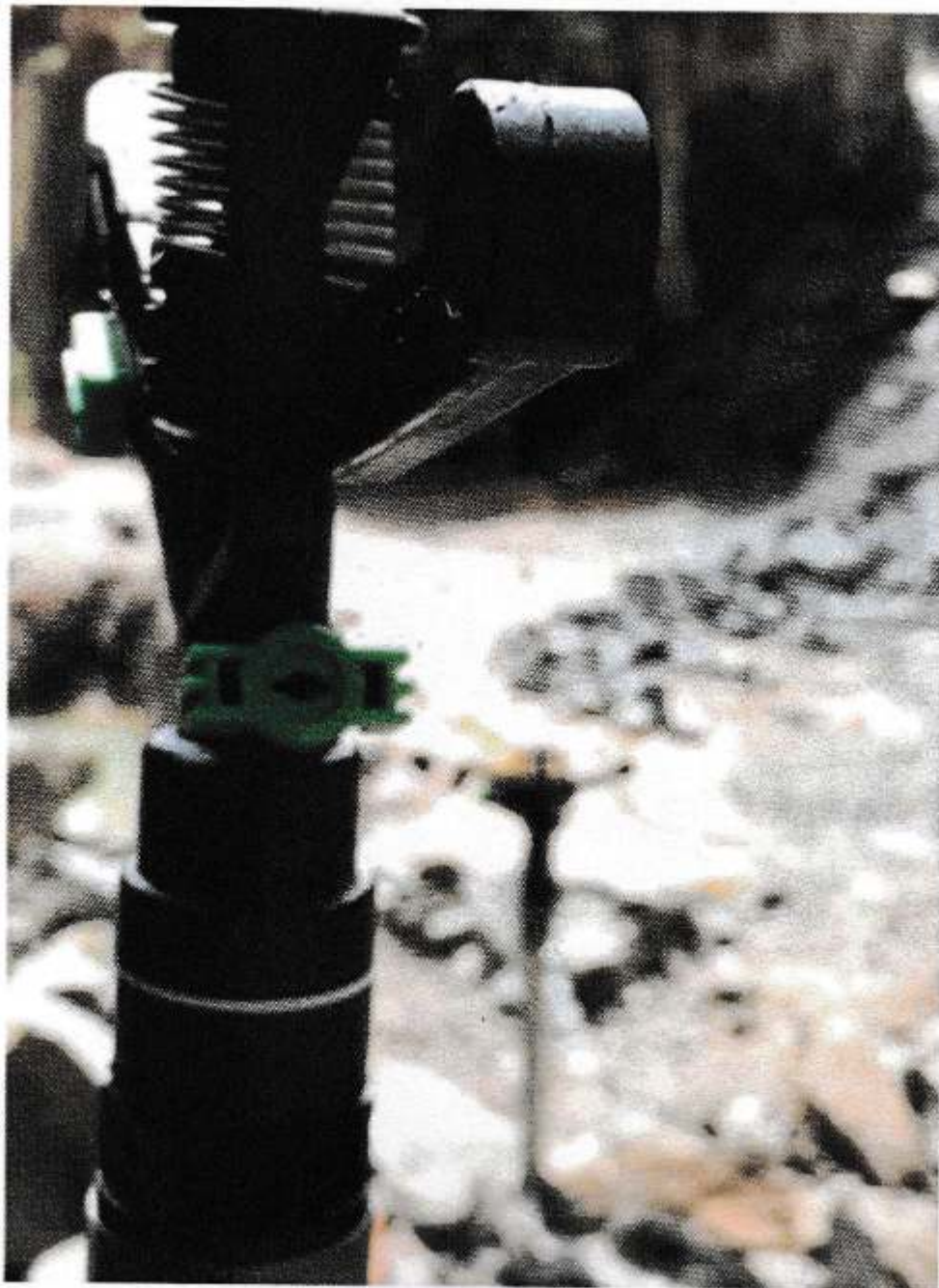
Plate S-10: Sprinklers
