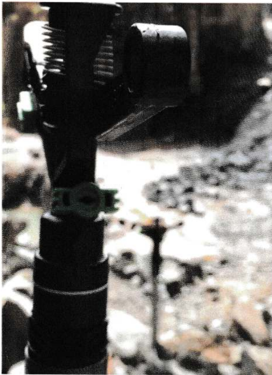
Plate G-5: Sprinklers
