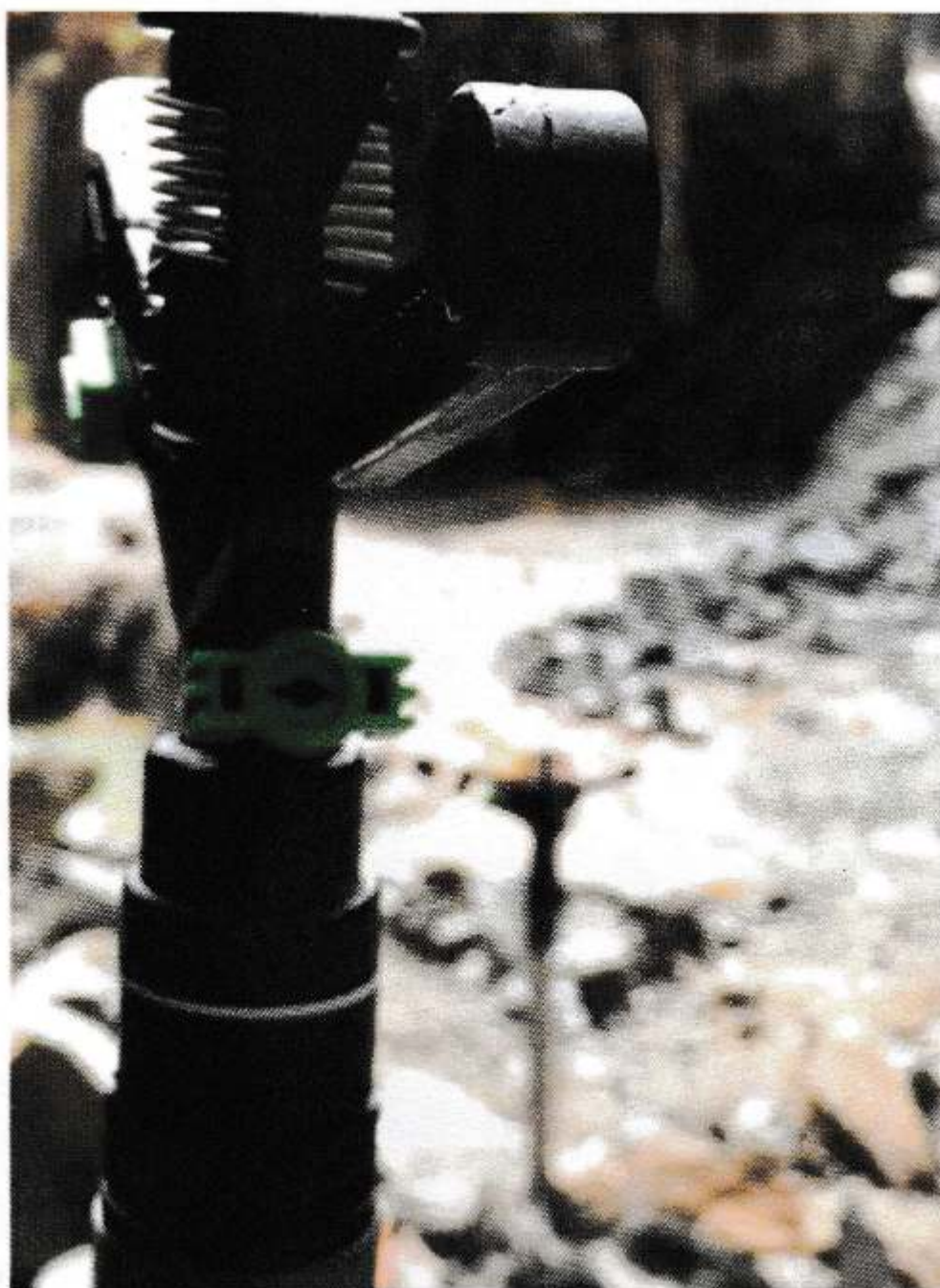
Plate S-10: Sprinklers
