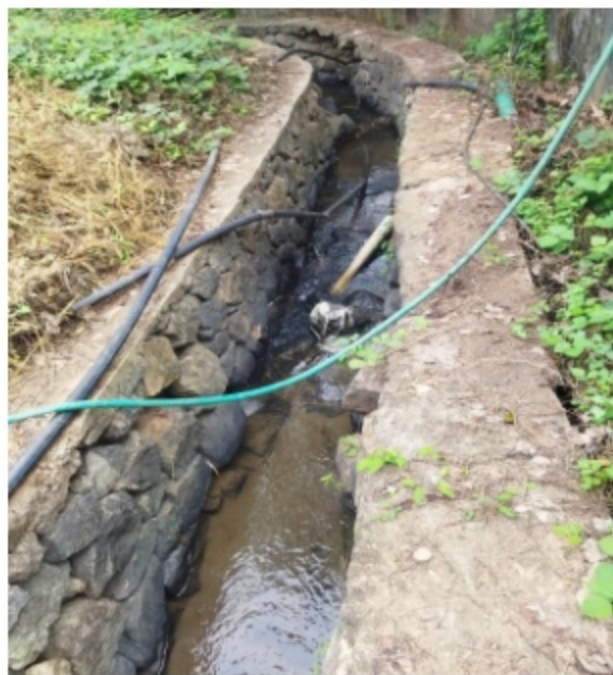
Fig 3: Photograph of drain leading to pond
